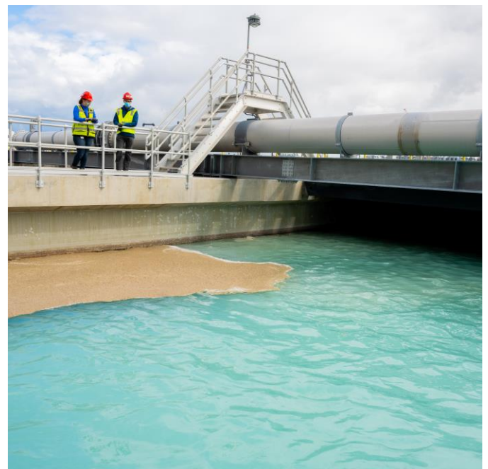
Water Recycling Facility at Intel's Gordon Moore Park at Ronler Acres Campus.
