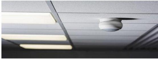
Security, environment control
